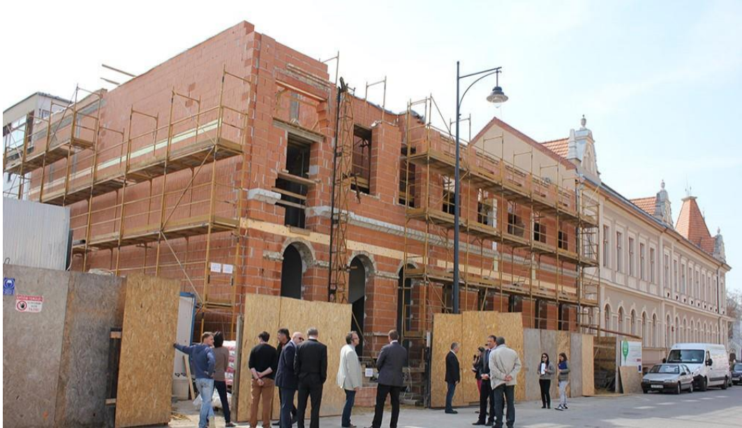
Photo 4 The Petöfi Street wing of the Hajdúböszörmény District Office (investment has been already finished) (Source: news.hajduboszormeny.hu)
